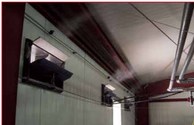
Figure 6.21: Example fogging system for a cross-ventilated house.
