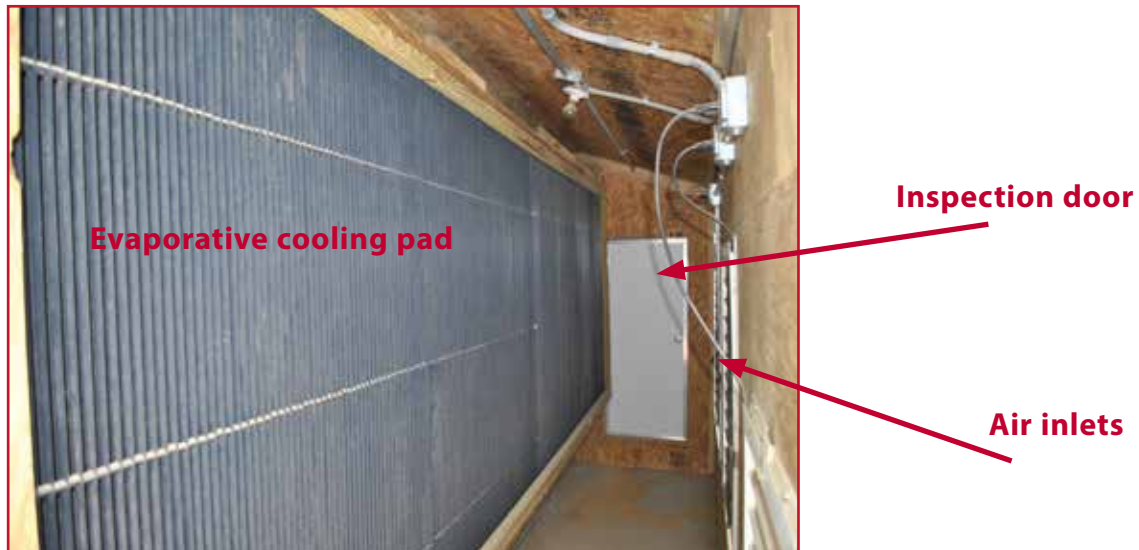
Figure 6.20: Example of a cooling pad installed on the sidewall of the house in a doghouse.
